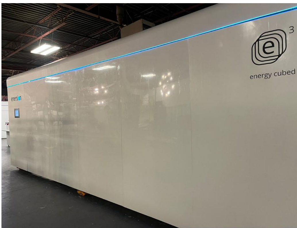
Figure 2: Photo of chiller
