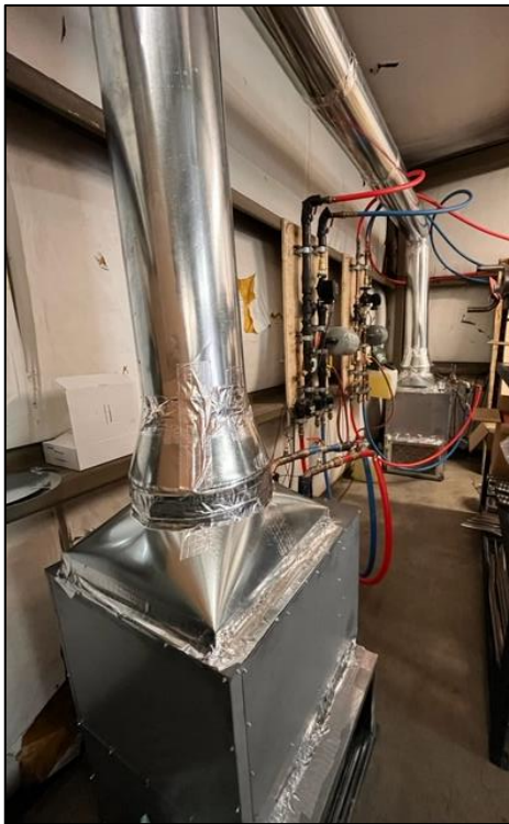
Figure 11: SMTI – Indoor Installation
