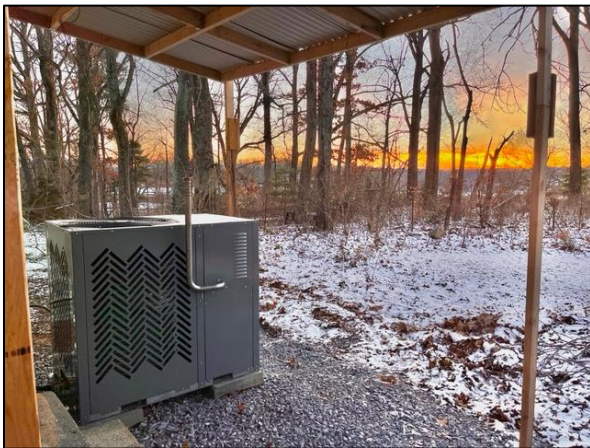
Figure 9: GAHP Life-Test Installation #1
