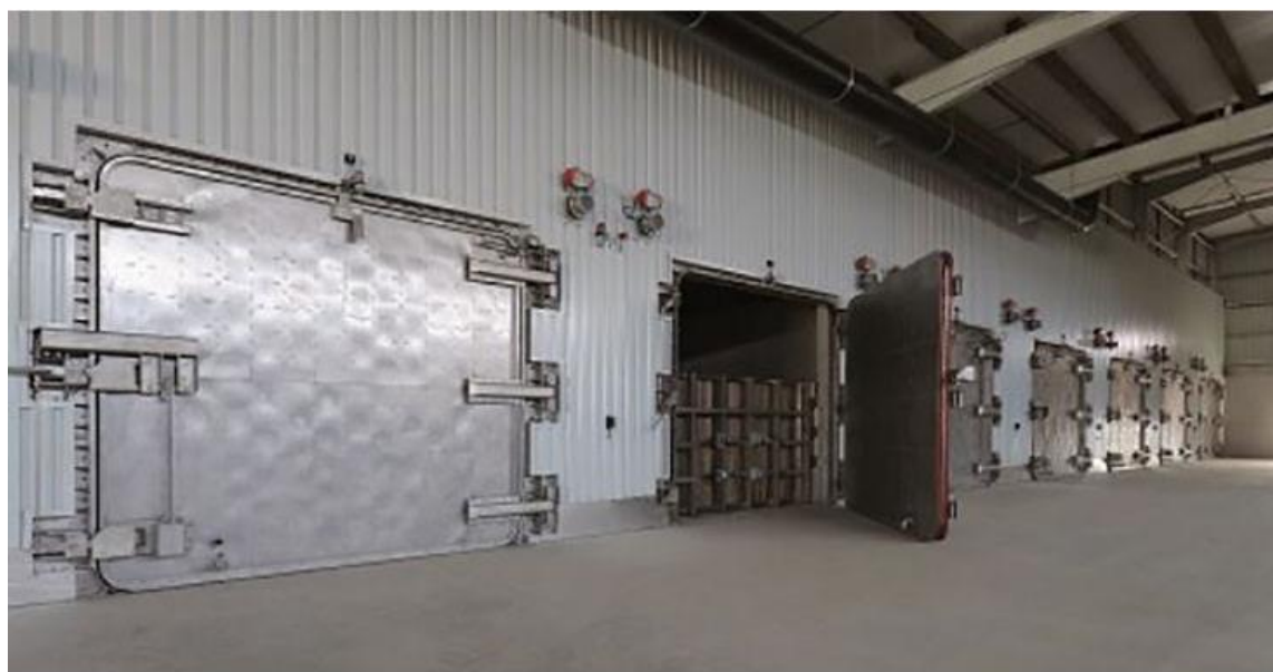
Figure 2.4: Overview of the HSADF digesters
