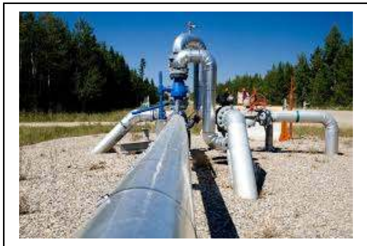
FIGURE 2-4. SIMULATED METHANE SOURCE: GAS-GATHERING PIPELINE
