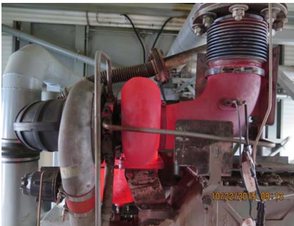
Engine Before REMVue Installation
