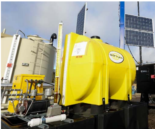
Solar Chemical Injection Pumps
