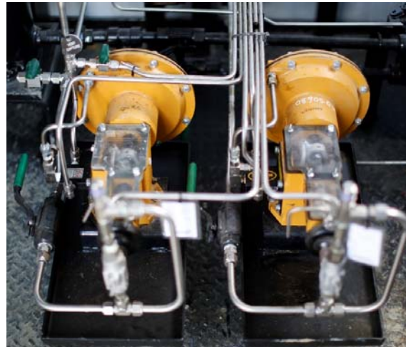
Pneumatic Chemical Injection Pumps
