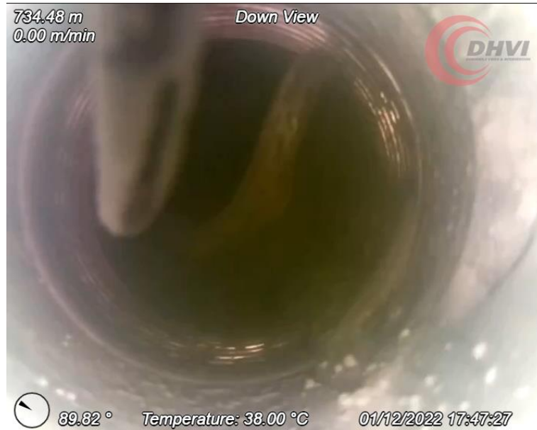
Figure 16- Leg 1 Image of Severed DTS Fiber at Latch
