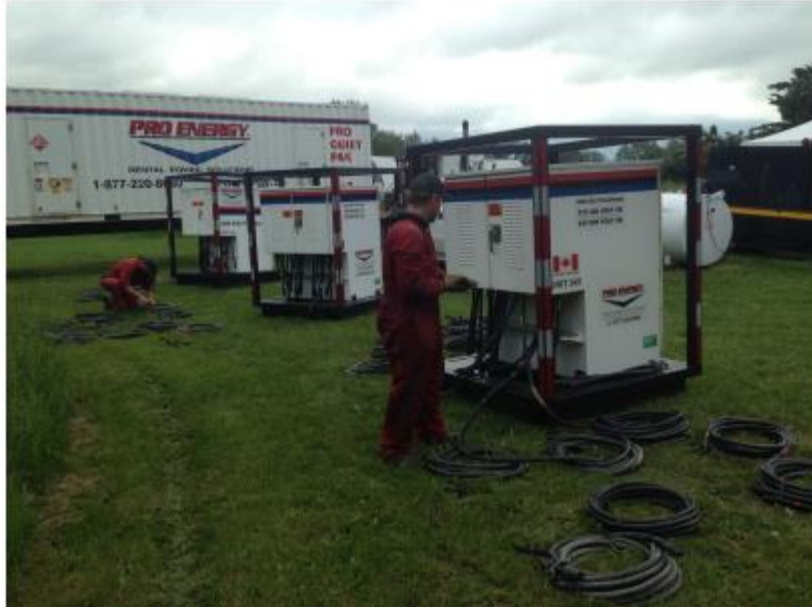
Figure 6- Diesel Generators with Transformers
