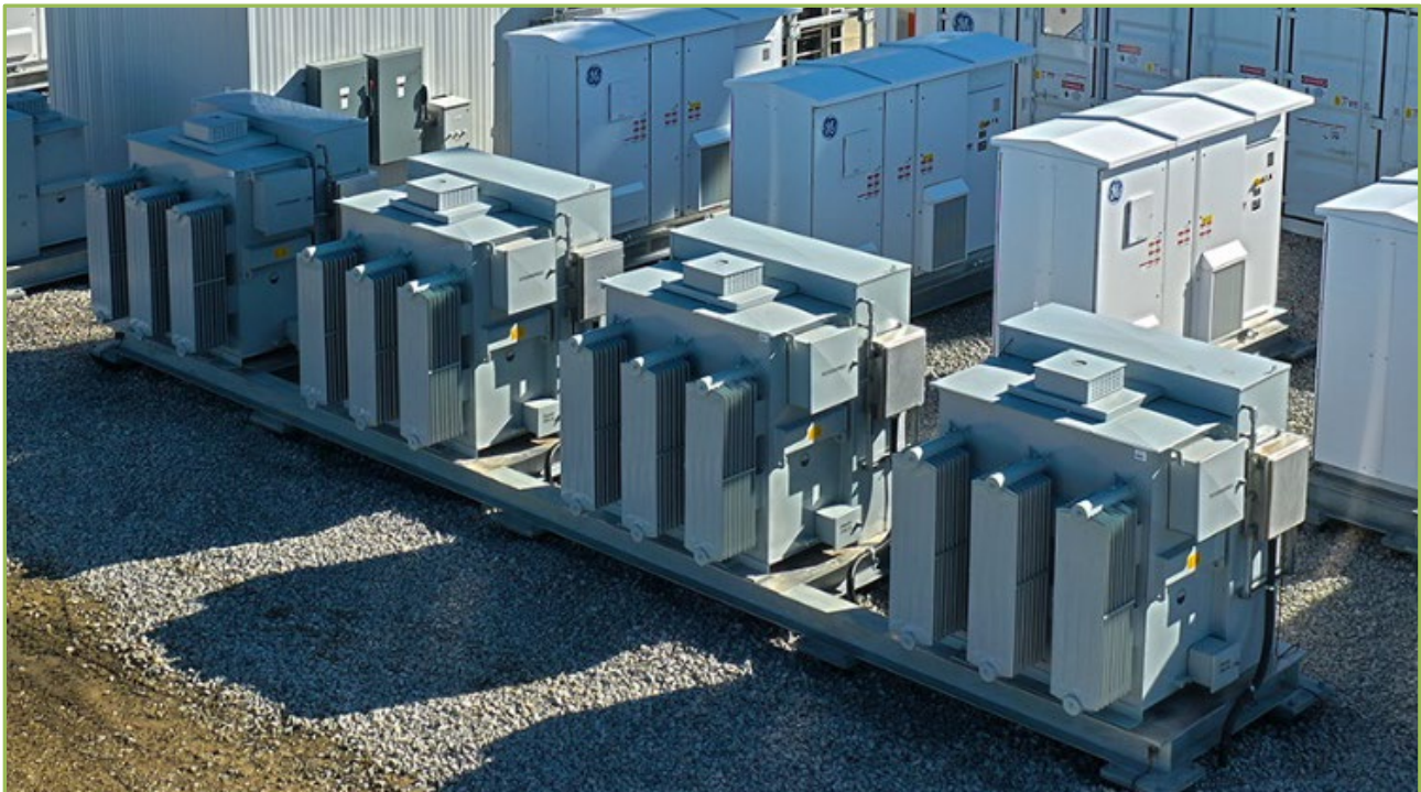
Picture of 4 of the transformers (there are 8 total)
