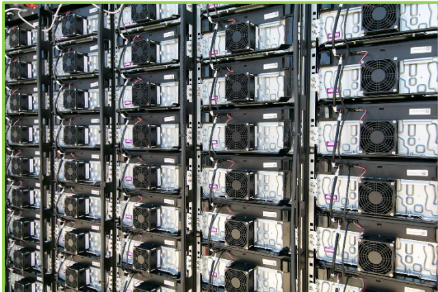
Picture of battery racks inside the HPSU
