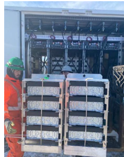
Battery Modules being loaded into HPSU
