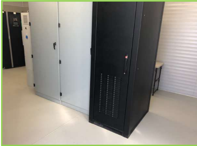
Picture of control cabinets inside the Control Enclosure Building
