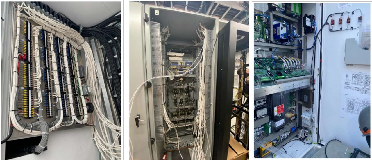
Interior of control cabinets within the BESS Control Enclosure
