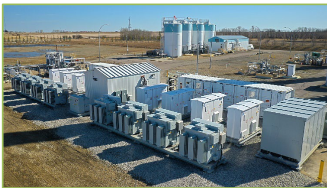
Picture of integrated BESS Components
