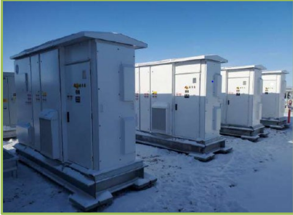
Picture of four inverters (there are 8 total)
