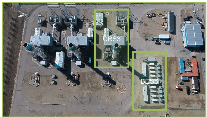
Aerial picture of Crossfield showing BESS with Turbines
