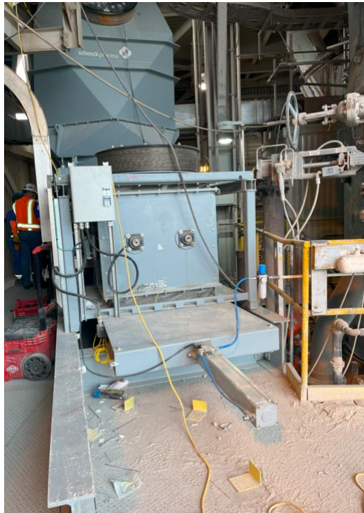
Figure 9 MultiFlex Dosing System - Precalciner
